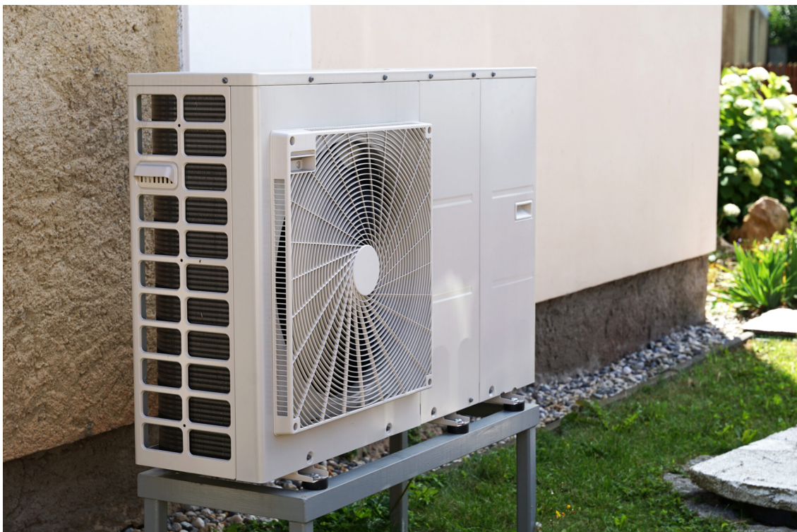
Boiler Upgrade Scheme
